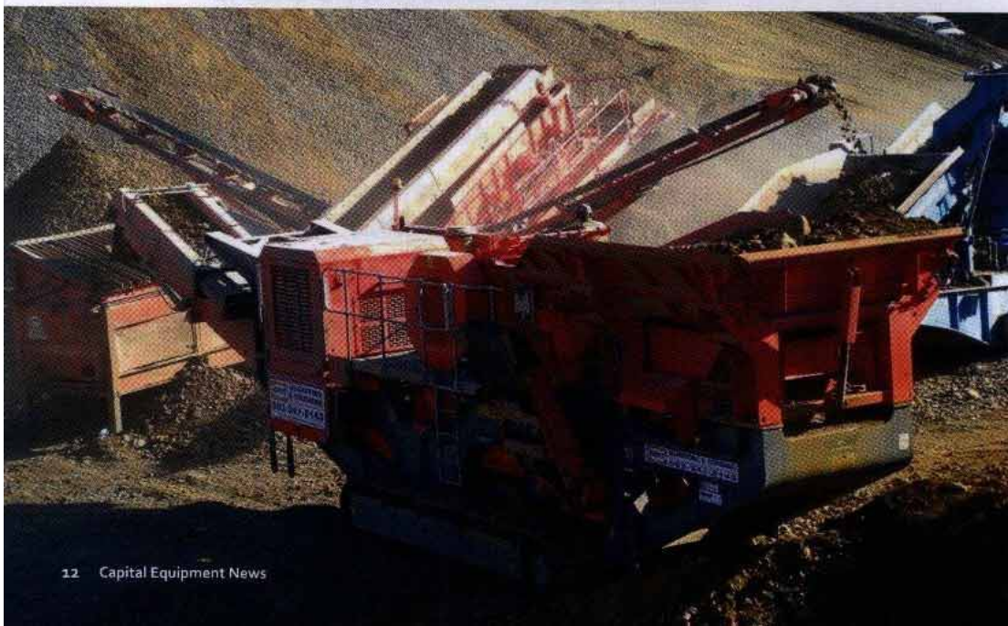
One of the borrow pits on the N17 with the Pilot Crushtec J-1175 jaw crusher in the foreground.
